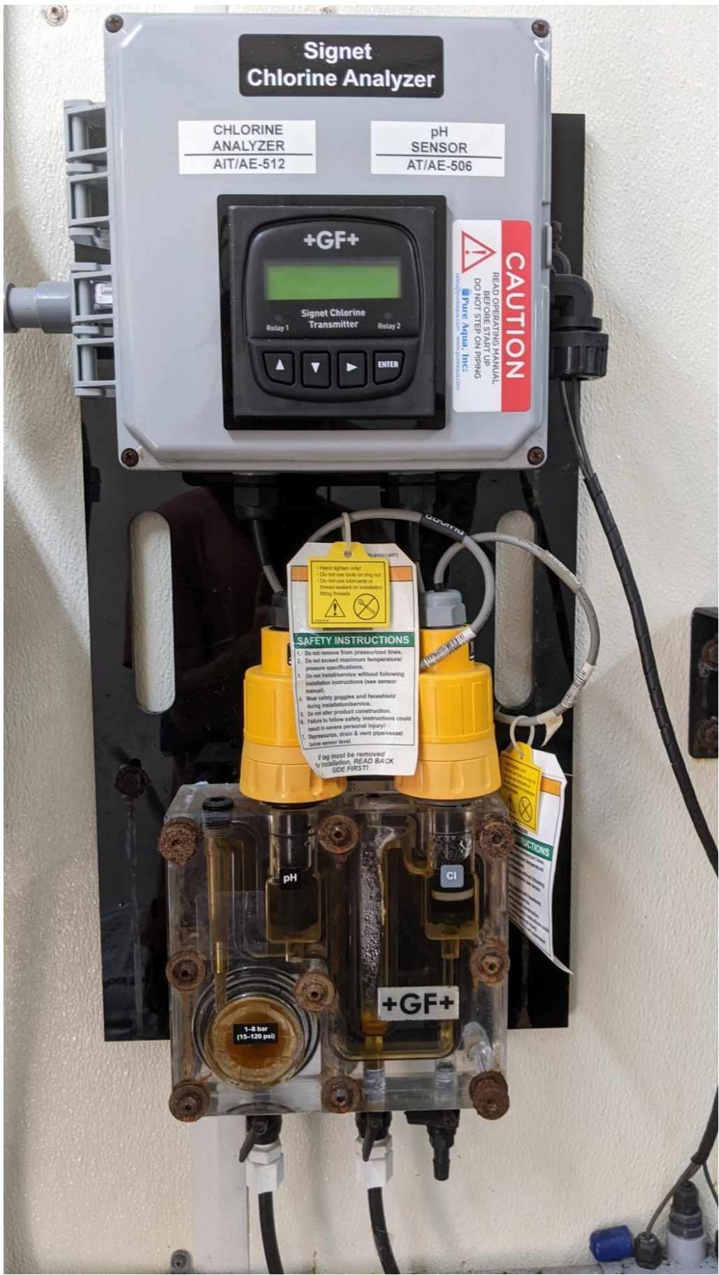
Figure 4. Faulty automatic chlorinator (GF Signet 4630 Chlorine Analyzer System)
