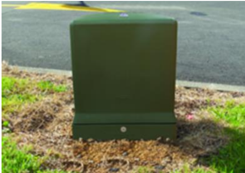
Figure 41. Example of a pillar box. Source: Transnet
