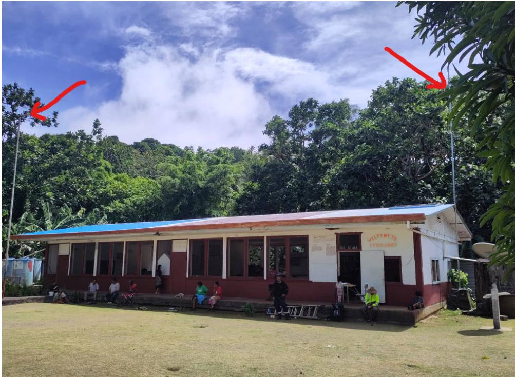
Figure 29. Antenna and standalone solar system on the roof of the school (left), pole in the plot of land (right)
