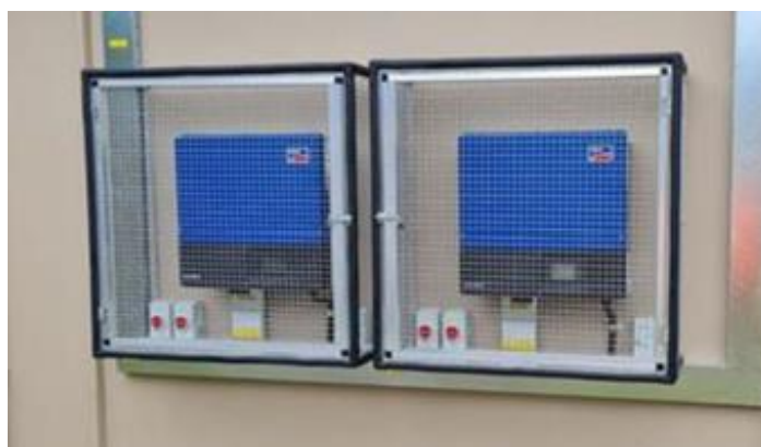
Figure 31. Example of a metallic cage that protects outdoor inverters from theft. Additional protections against water should be considered also
