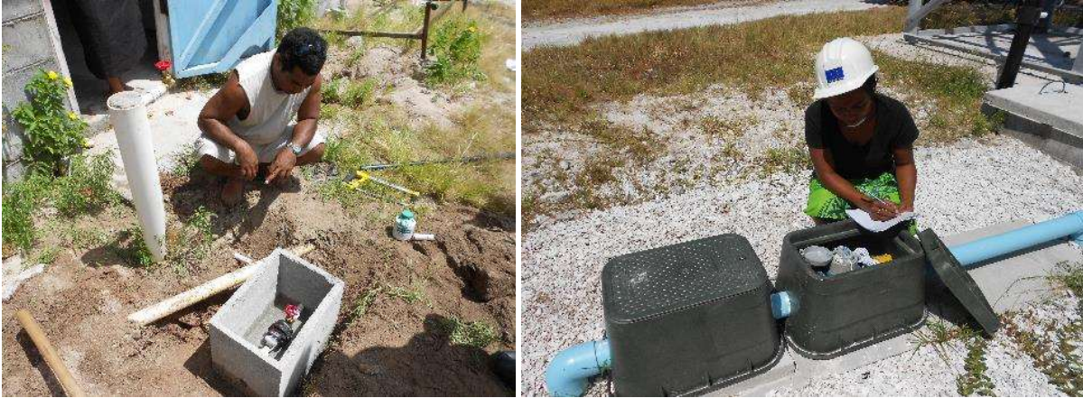
Figure 21. Household water meter installation (left) and pump well bulk flowmeter (right)
