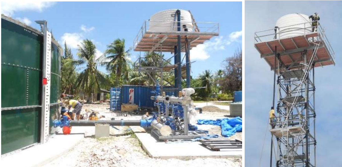
Figure 19. London water storage (left) and Decca header tank (right)
