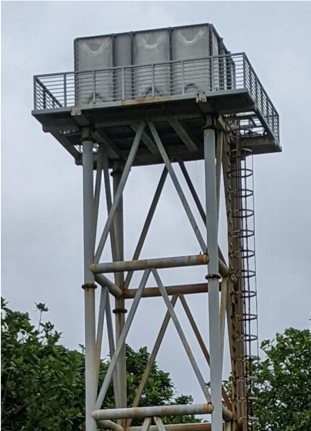
Overhead storage tank near catchment area requiring flooring and ladder repairs.
