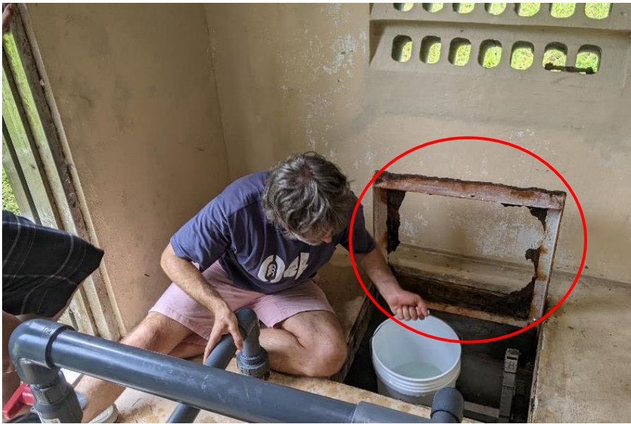
Well lid in pump house requiring replacement.
