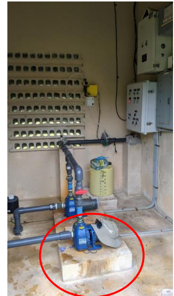
Pump base requiring elevation.
