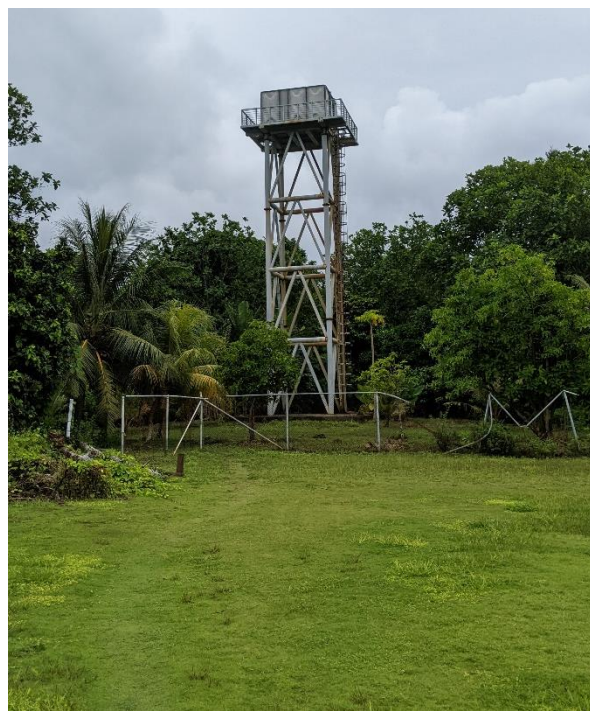
Overhead storage tank near catchment area requiring flooring and ladder repairs.
