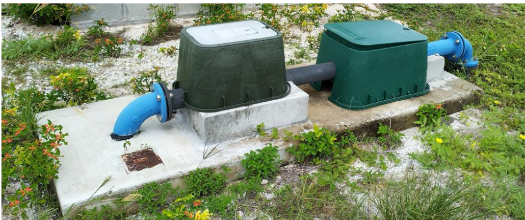
Figure 24. Example 80mm flowmeter and slab installation at Decca lens
