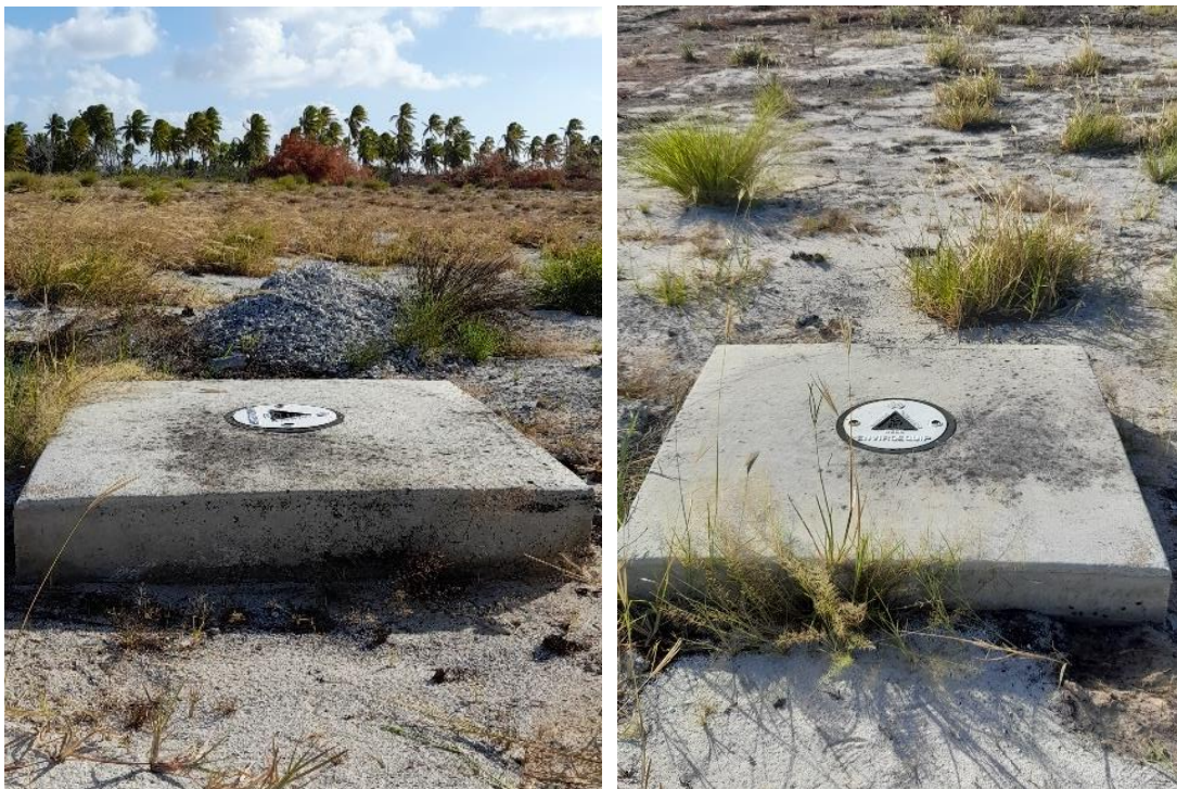
Figure 26: End gallery cover at Decca gallery 6 installed in the previous project
