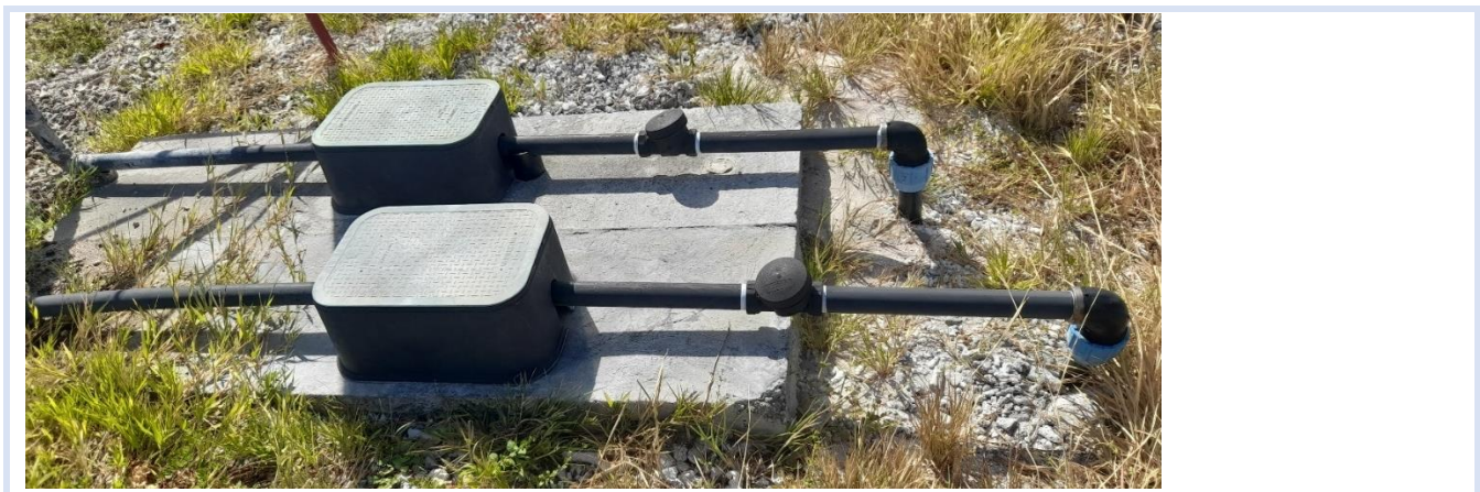
Figure 22: Flowmeter concrete slab at Four Well pump well
