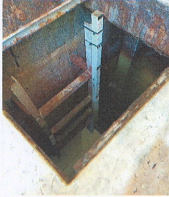
Wet Well Tank – 1 piece (Control low level)
