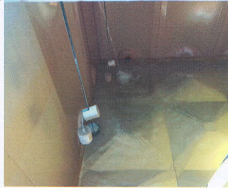
Elevated Tank – 2 pieces (Control low and high level)
