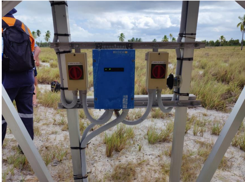
Pump Control Unit
