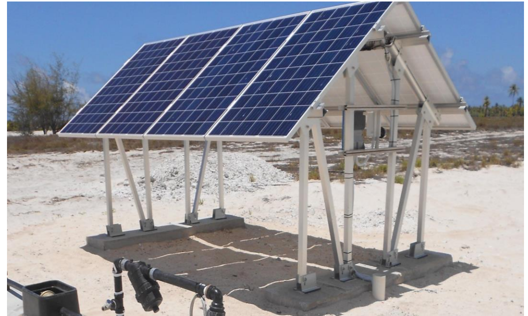
Solar Panel Array
