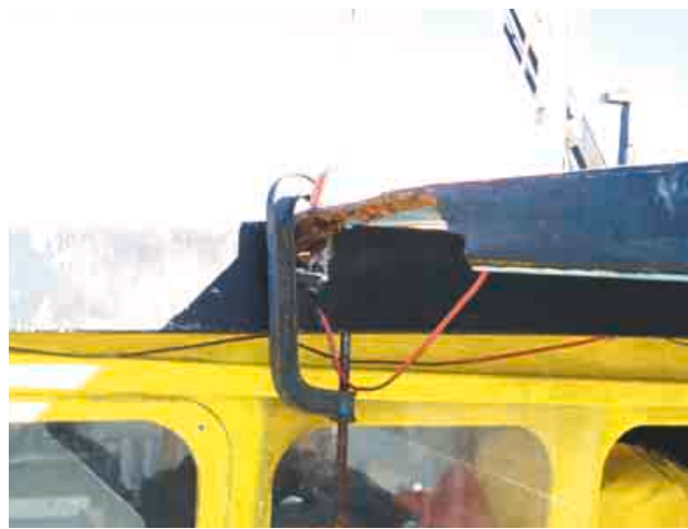
Figure 14: Evidence of dry rot in the sunroof.
