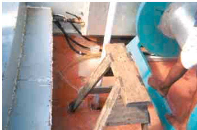
Figure 13: Water accumulating on flat deck
