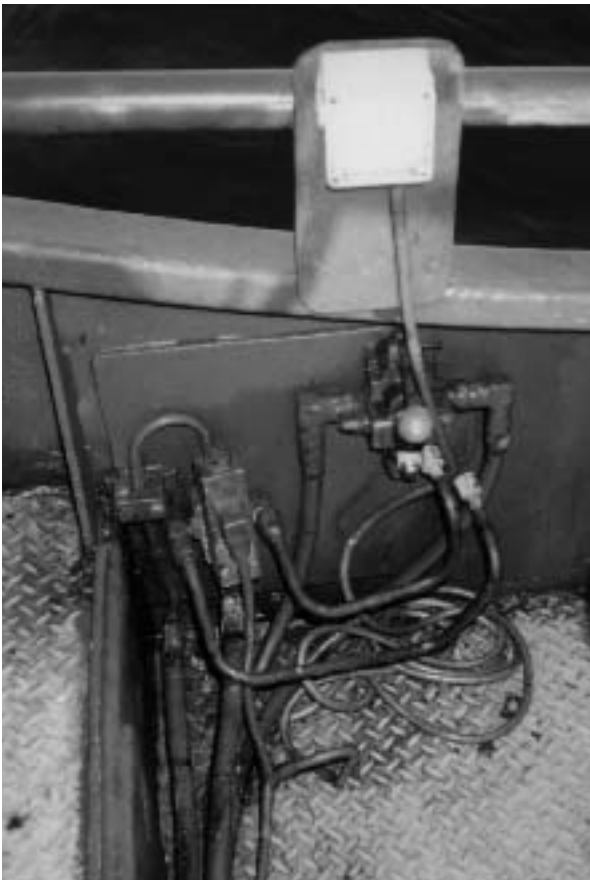
Figure 13: 'Brand' hydraulic valve with electric solenoid by-pass valve
