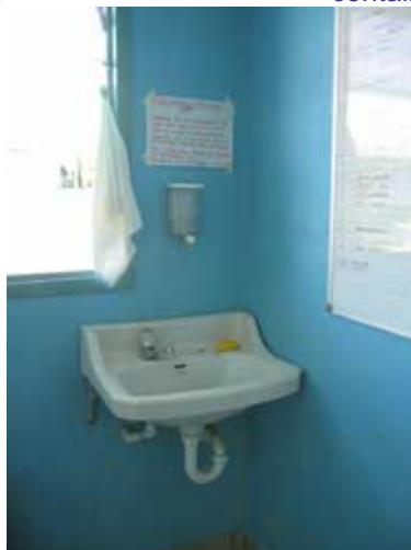
Basic hygiene facilities at point of use help staff comply with hand hygiene practices.
