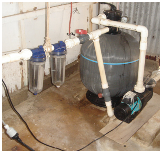
Water filtration system in a quarantine area
