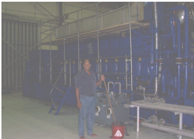
Figure 5: UNELCO 4 MW diesel Genset in Port Vila
