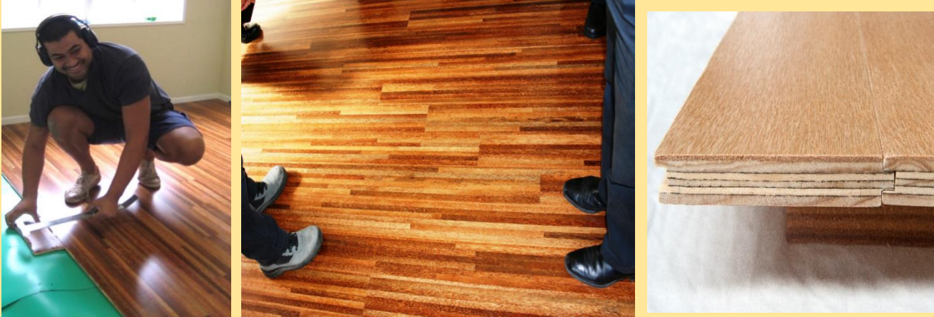
Fig. 3. Engineered cocowood T&G flooring combining sawn coconut wood and plywood being installed.
