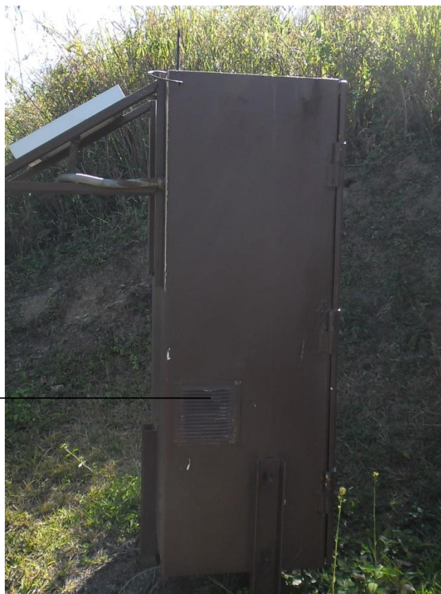
Figure 9 Grille de ventilation
