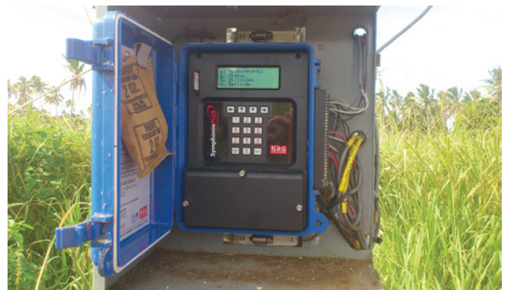
Data logger for recording wind measurements at the bottom of the Lapaha wind monitoring mast, photo: Kevin Palmer-Wilson, GIZ
